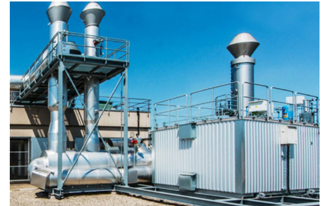
Once the Oxi.X RV exhaust-air purification system has reached its operating temperature, it is energetically self-sustaining.
