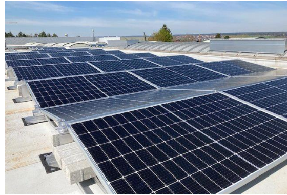
10| Photovoltaic systems in Holzbronn (Germany) (Source: Dürr AG)
